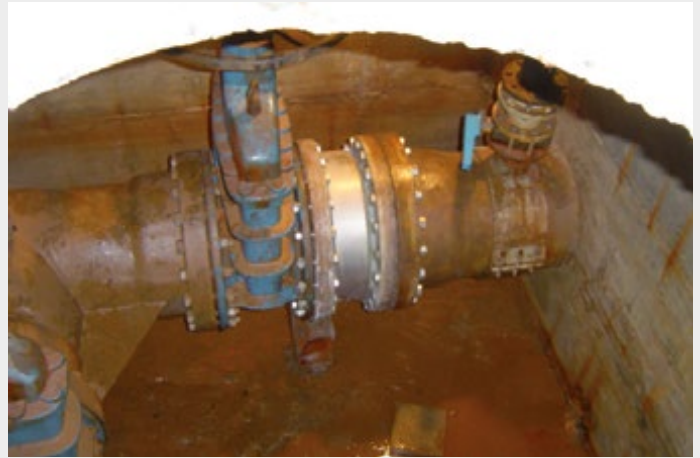
Installation within a distribution chamber.
