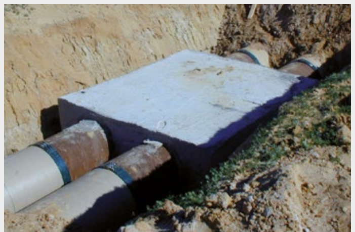
Connection of GFP and steel pipe with different outer diameters at the inlets and outlets of a distribution chamber.
