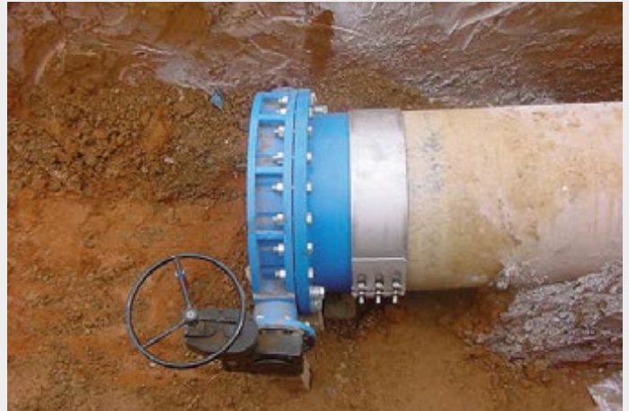
Connection of a GRP pipe with a shut-off valve.
