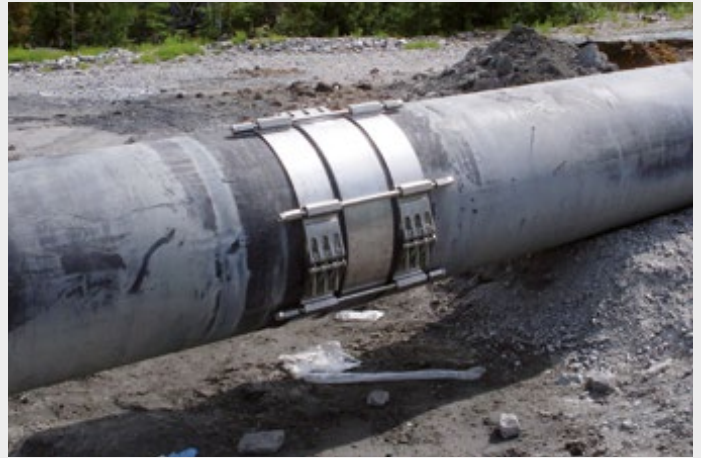
Tensile-resistant installation of a PE pipeline for the waste water of a mine.
