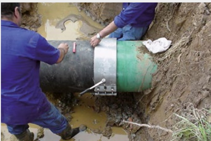
Repair of a GFP pipe with a pipe section made of cast iron with different outer diameters.
